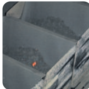
Hot clinker conveyor
